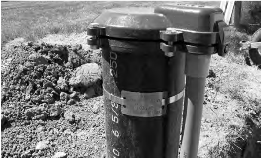
A well tag, displaying the well identification (ID) number, should be on every well.
