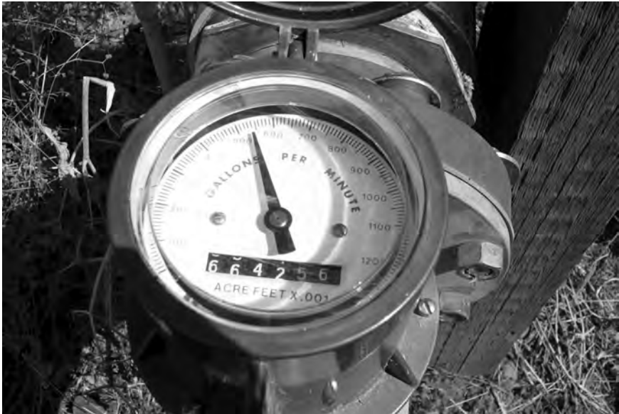
This photo is an example of a water meter device.
