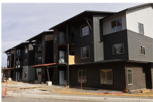
The Shiloh Crossing affordable housing apartments under construction at the south end of Bend in October 2021.
